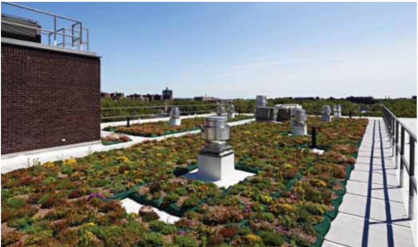
Green roof on permanent affordable housing in Brownsville, Brooklyn.
